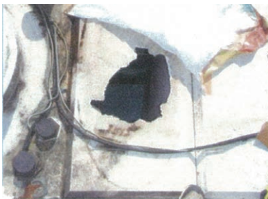
Deterioration over time
